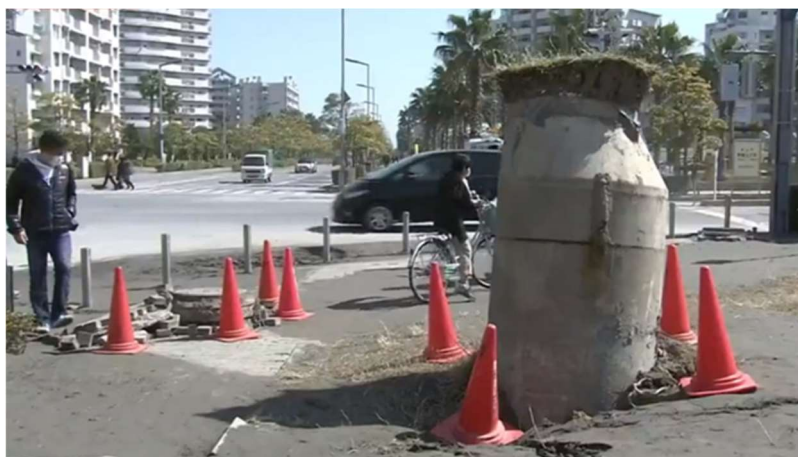
Figure 3. Sewage manhole that broke out on the surface due to the liquefaction, Abiko city in Japan
