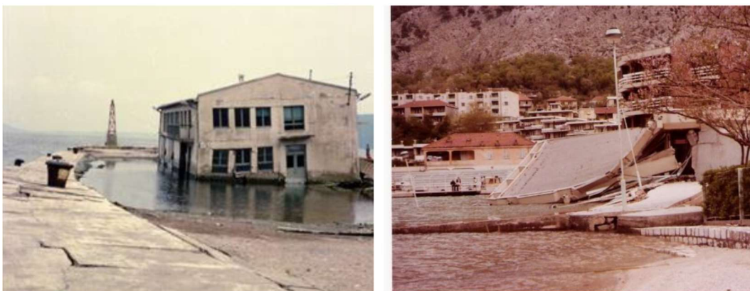
Figure 2. Subsidence of the terrain under the warehouse in the port of Zelenika, left picture; Heavy damage to Hotel Fjord – Kotor city, right picture
